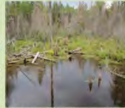
Water ponded upstream of an old crossing is a good indication that the crossing is set too high.
